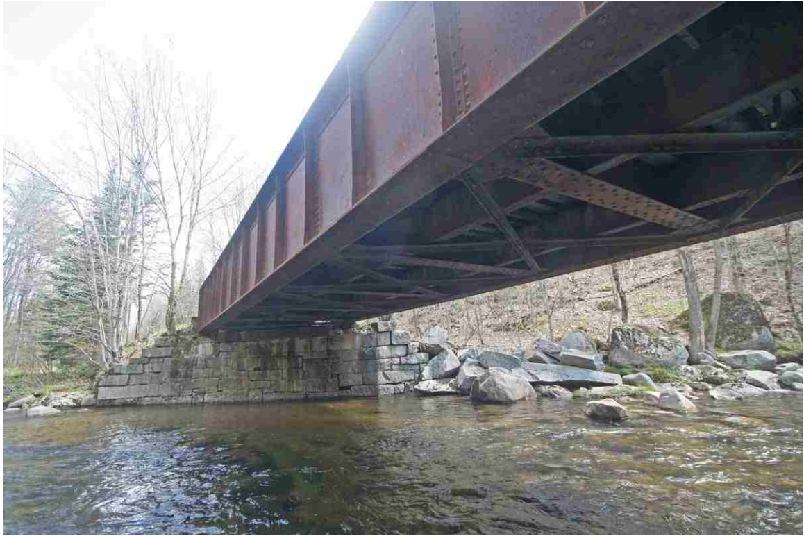
Photo # 95 description: Bridge 145.73, Gorham, "Moose River Bridge No. 2." Underside and east abutment. (4 of 4).
