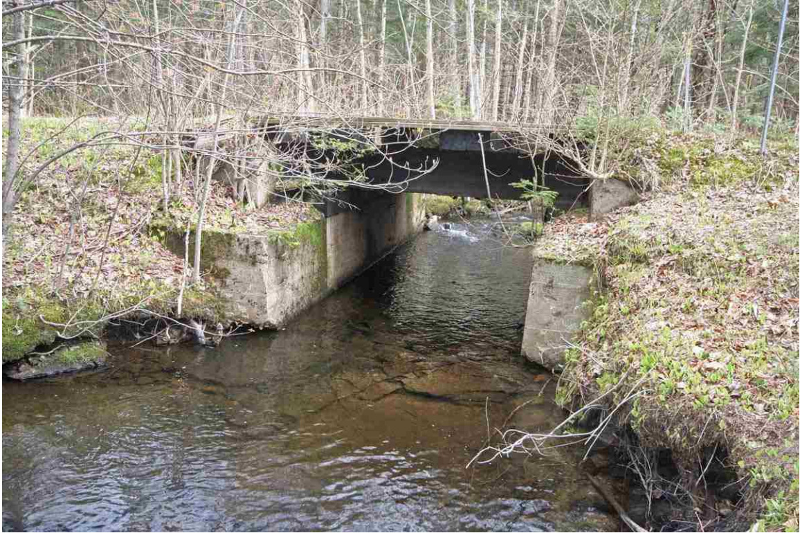
Photo # 49 description: Bridge 140.50 over Moose R., Randolph. Wood stringer, 7' span, on concrete abutments. Downstream side. 1923, 1943.
