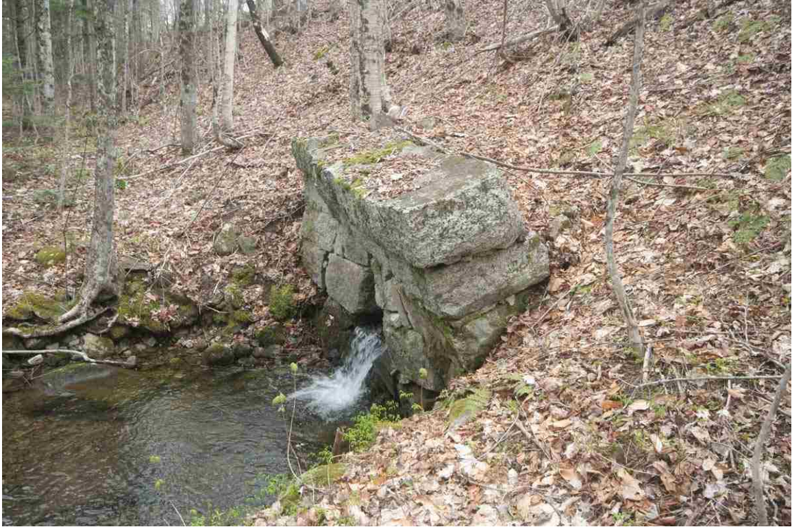
Photo # 57 description: Culvert 142.19, Randolph. (2 of 2). Critical condition; collapse imminent.
