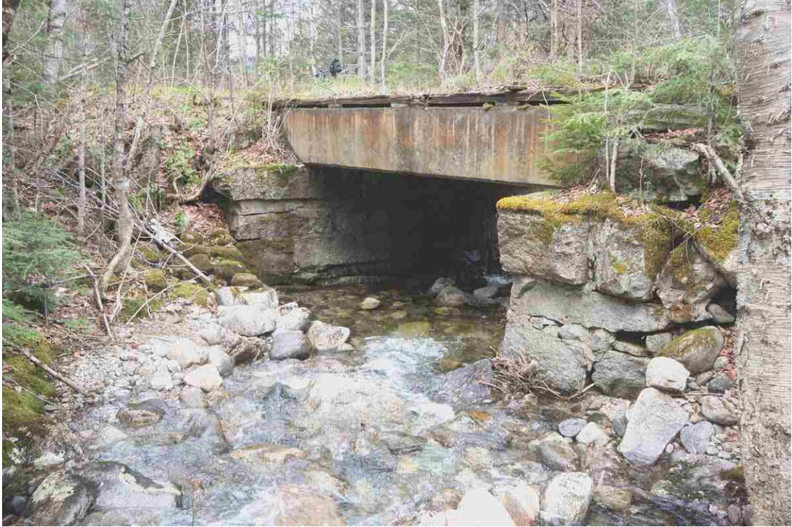
Photo # 83 description: Bridge No. 145.09 over Town Line Brook, Randolph-Gorham. Precast concrete slab on mixed split quarry & fieldstone abutments, 14-0 span. 1930. Upstream side. (1 of 2).
