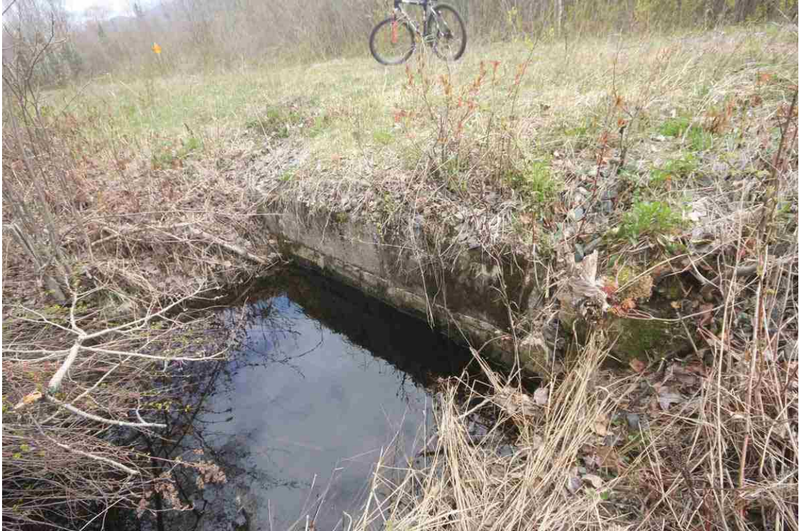
Photo # 23 description: Culvert 134.81, Jefferson. Stone box retrofit with 12" cast iron pipe, underwater. nd.
