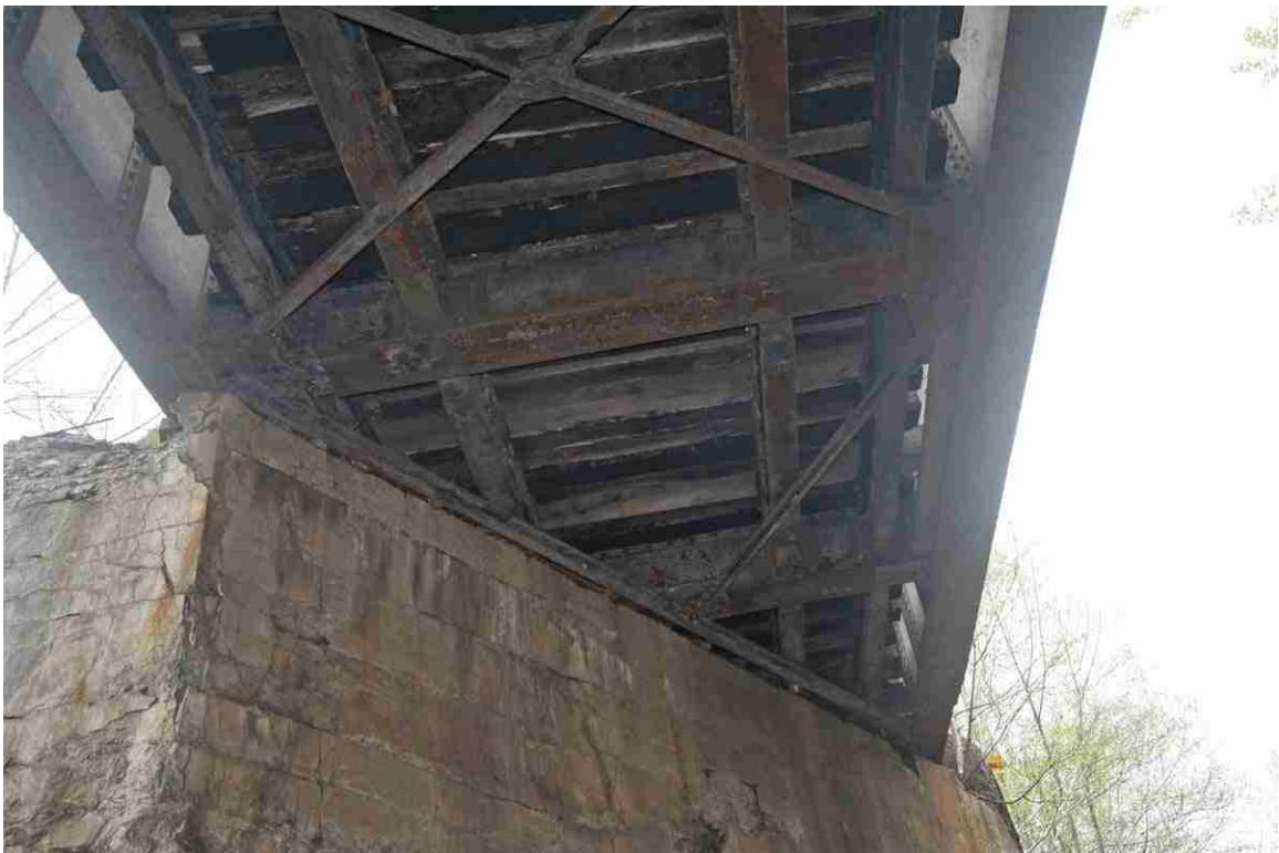
Photo # 132 description: Bridge 153.14 over A&SLRR at Berlin Mills Station, Berlin. Underside showing framing and ties still in place under new deck and gravel fill. Both abutments deteriorating.
