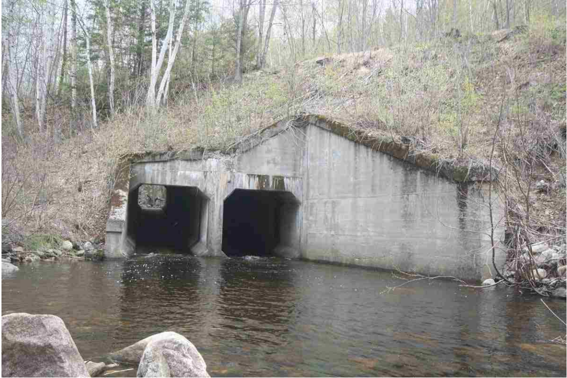
Photo # 127 description: Culvert 152.49, carrying Cascade Alpine Brook, Gorham. Double 10' concrete box with 44' of cover. 1940. Major structure.
