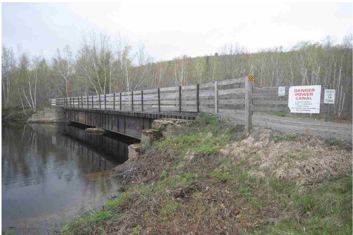
Photo # 120 description: Bridge 149.71 over Berlin Mills power canal, Gorham. Deck plate girder, 2-span, 87' overall, on concrete abutments. 1940. South approach and west side. (1 of 2)
