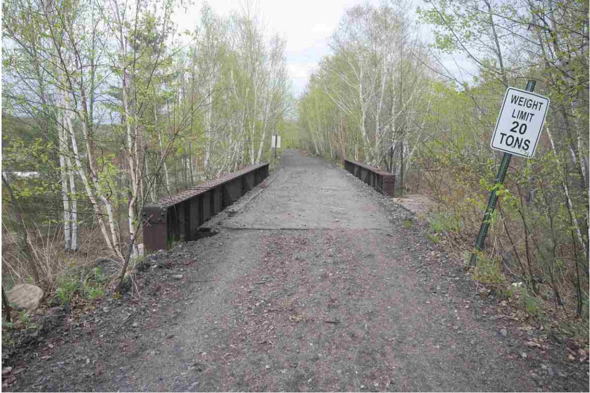
Photo # 129 description: Bridge 153.14 over A&SLRR at Berlin Mills Station, Berlin. Thru plate girder, 35' span, sharply skewed, on concrete abutments. 1940. South approach. (1 of 4).
