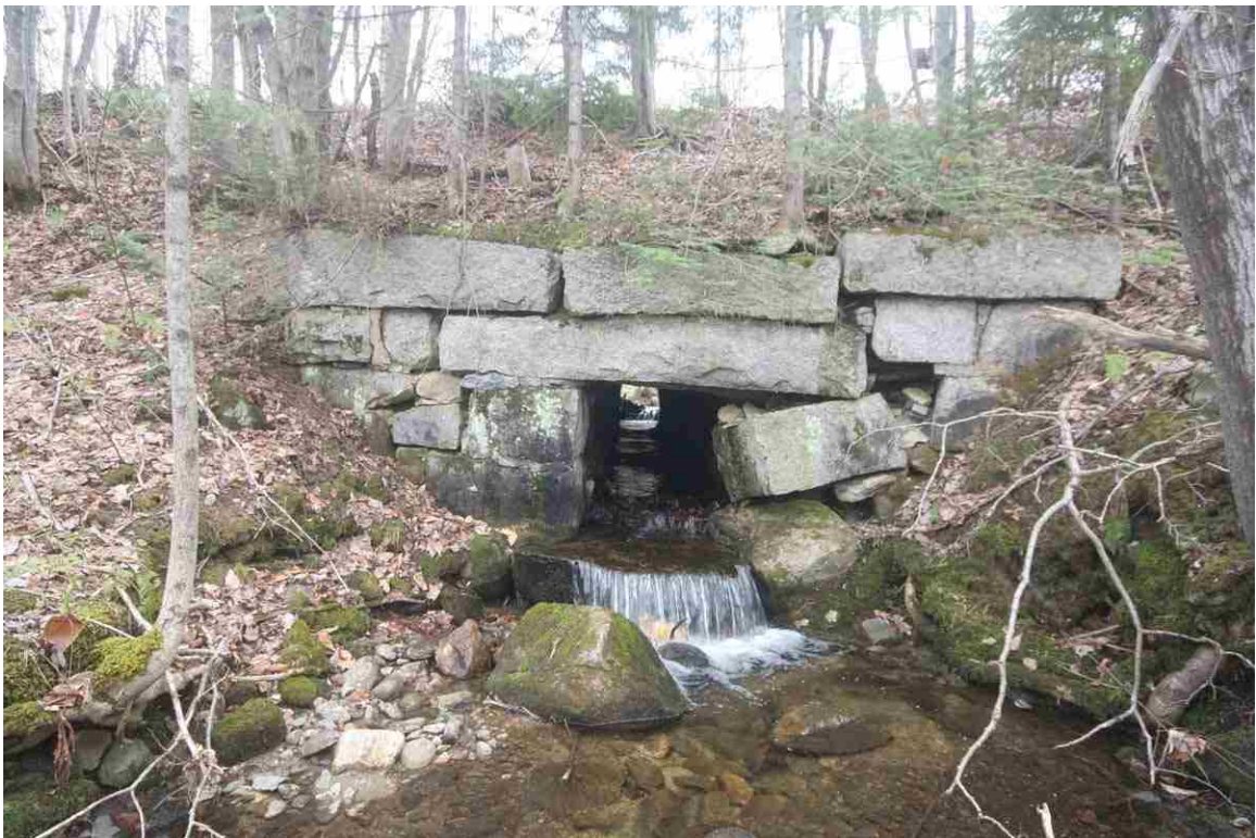
Photo # 64 description: Culvert 142.59, Randolph. Stone box, 54", mixed split quarry & fieldstone. nd. Note outlet headwall collapsing, condition critical.
