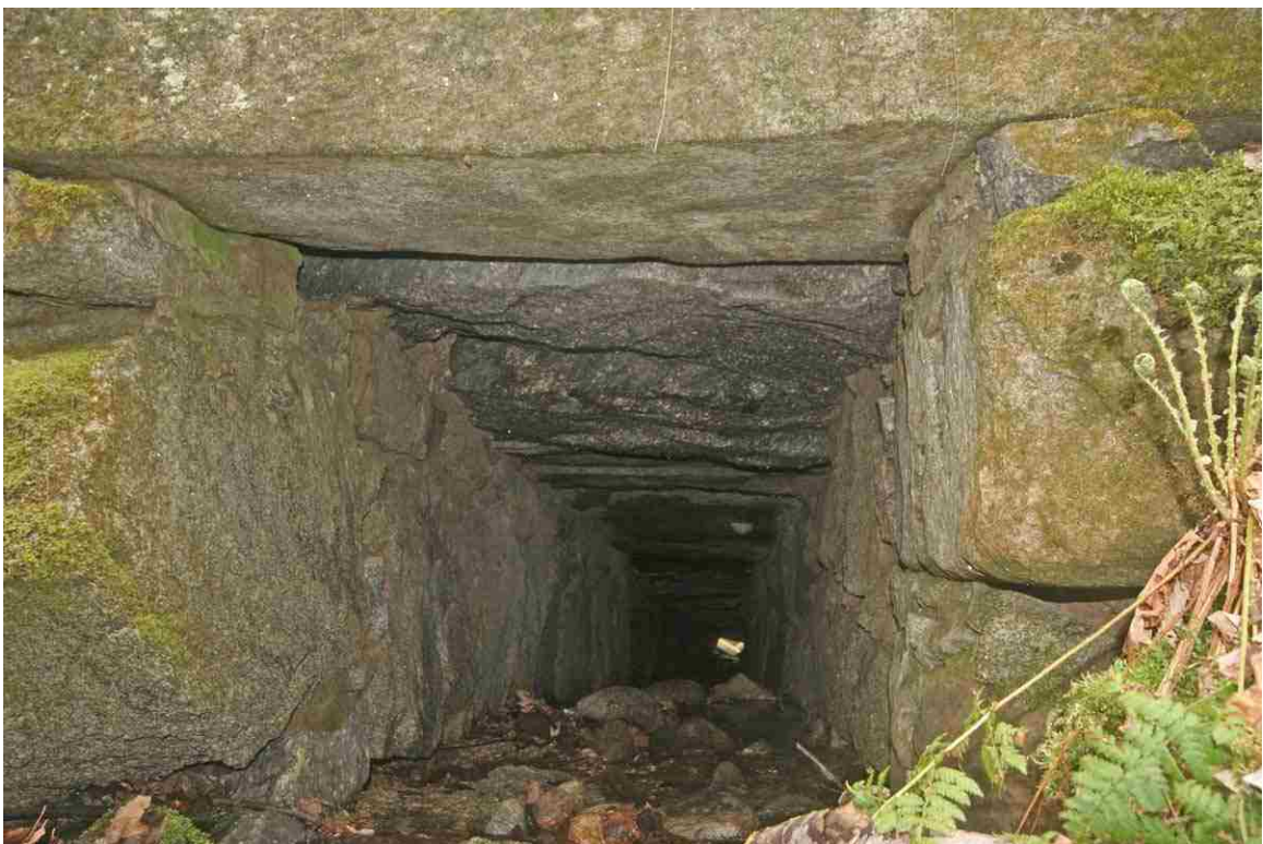
Photo # 102 description: Culvert 146.68, Gorham. Interior view. Exceptional length due to depth of cover; inlet opening just visible. (2 of 2).
