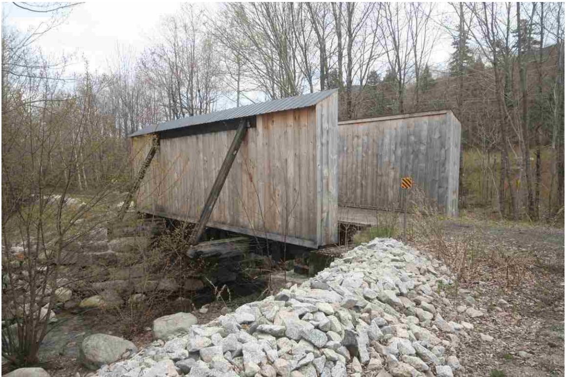
Photo # 66 description: Bridge 143.06 over Snyder Brook, Randolph. Pony Howe truss, boxed, 29' span, on rehabbed stone abutments. 1918. West approach and downstream side. (1 of 3).
