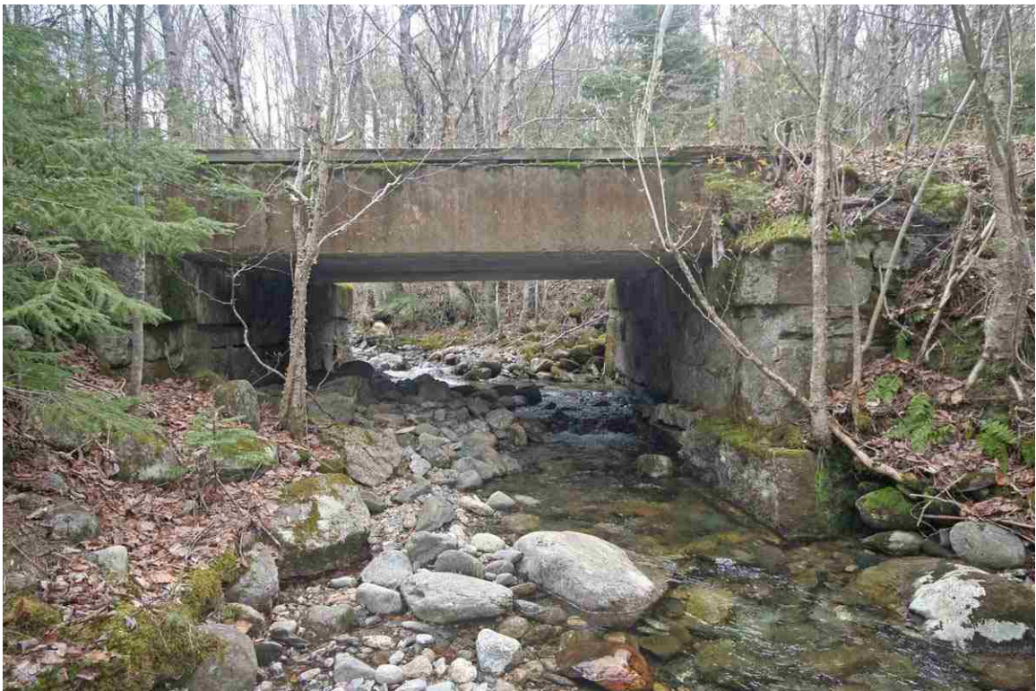
Photo # 84 description: Bridge No. 145.09 over Town Line Brook, Randolph-Gorham. Downstream side. (2 of 2).
