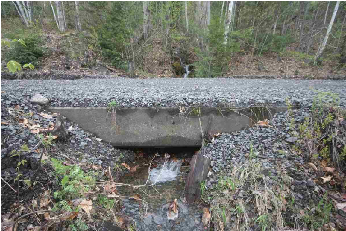
Photo # 122 description: Bridge 150.29, Gorham, over unnamed stream. Precast concrete slab on unknown substructure. 1930. Listed as 10' span in B&M bridge list.
