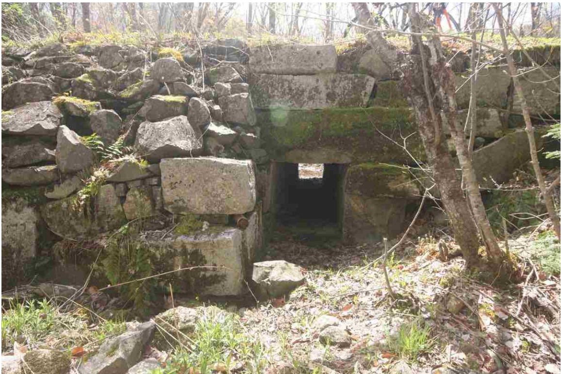
Photo # 90 description: Culvert 145.51, Gorham. Stone box, 36", mixed split quarry & fieldstone. Outlet wall partly reconstructed at left. (2 of 3).
