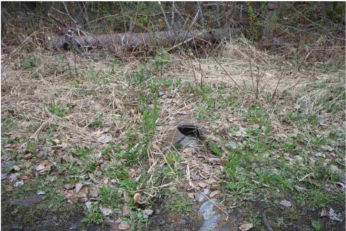
Photo # 40 description: Culvert 138.34, Randolph. Cast iron pipe, 24", with corrugated metal pipe inside. nd.
