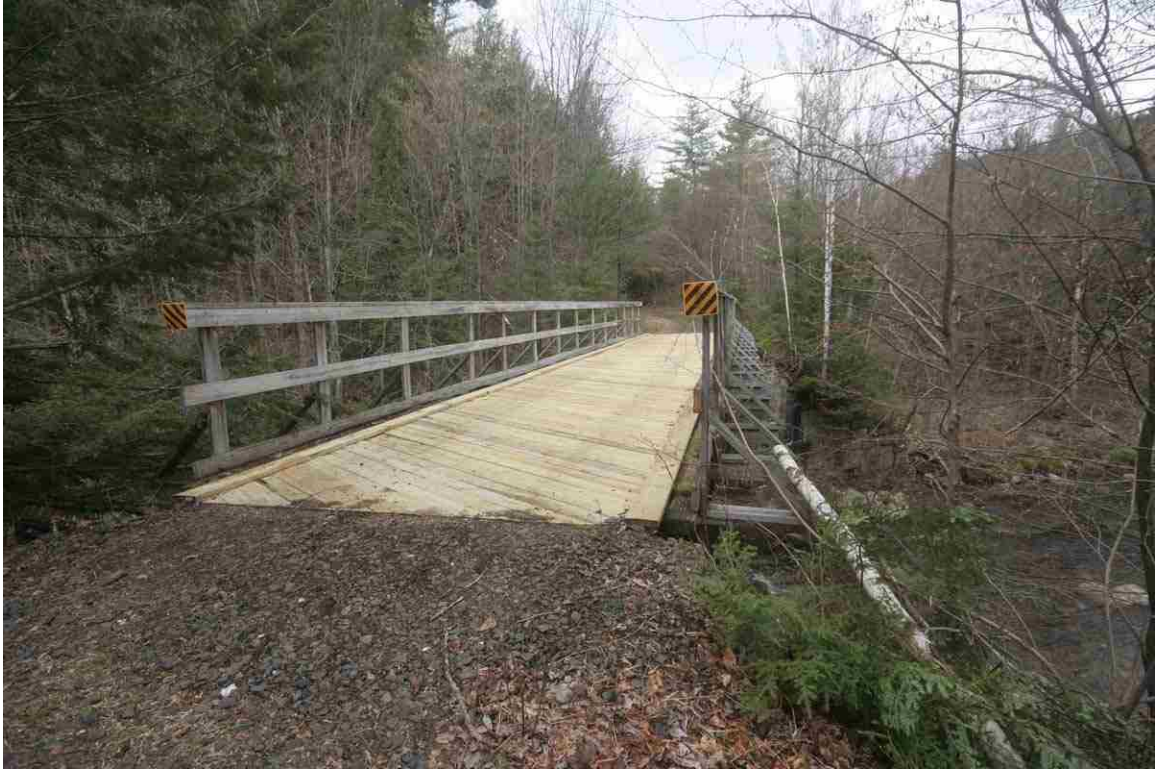
Photo # 103 description: Bridge 146.80, Gorham, "Moose River Bridge No. 3." Steel deck plate girder, 64' span on stone abutments. 1917. West approach. (1 of 4).
