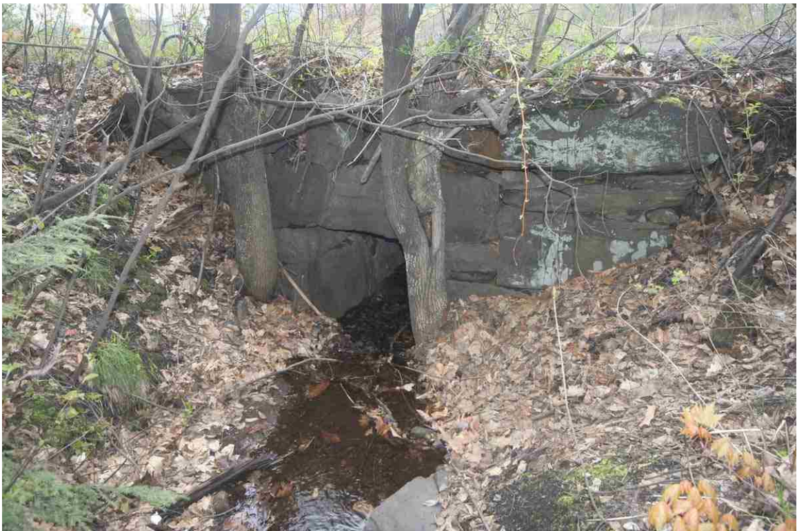
Photo # 128 description: Culvert 152.99, Berlin. Stone box, 36", mixed split quarry and field stone. Inlet. nd. Outlet repaired/extended with CMP.
