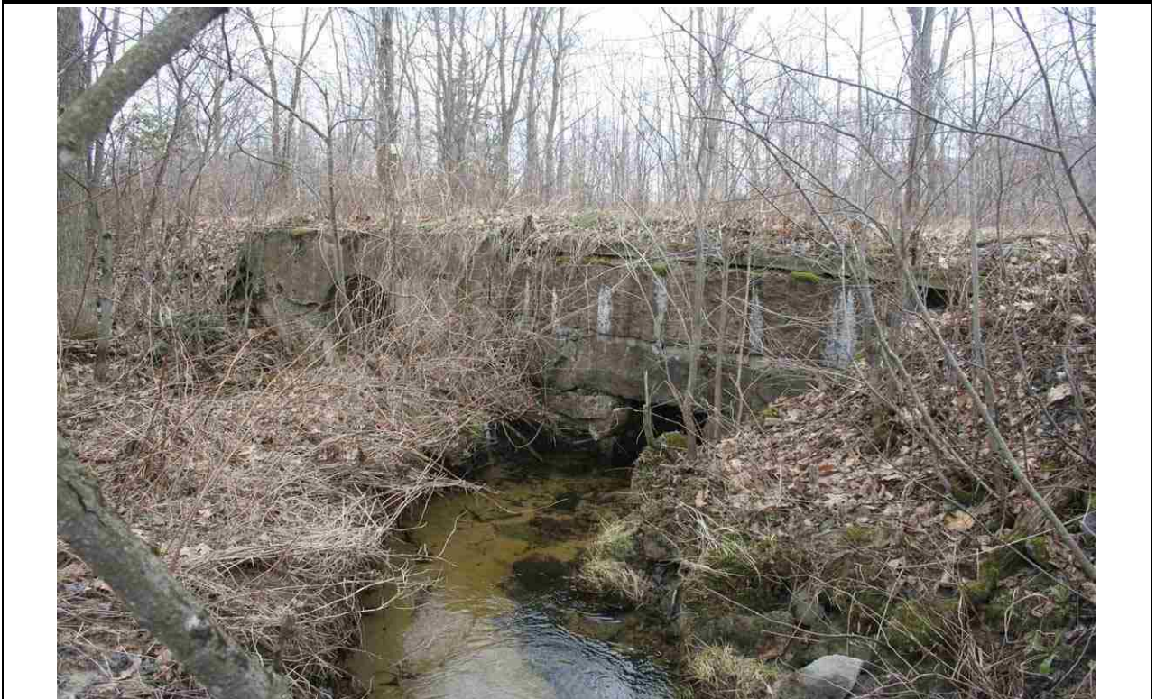
Photo # 26 description: Culvert 135.08, Jefferson. Stone box, 36". nd. Concrete pipe w/ concrete headwalls relief culvert added alongside. nd. (1 of 3).
