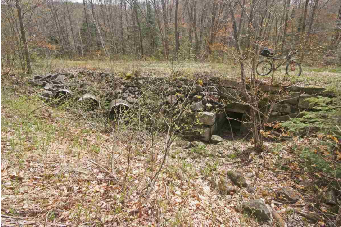
Photo # 89 description: Culvert 145.51, Gorham. Stone box and three later added CMP relief pipes, overall view. nd. (1 of 3).
