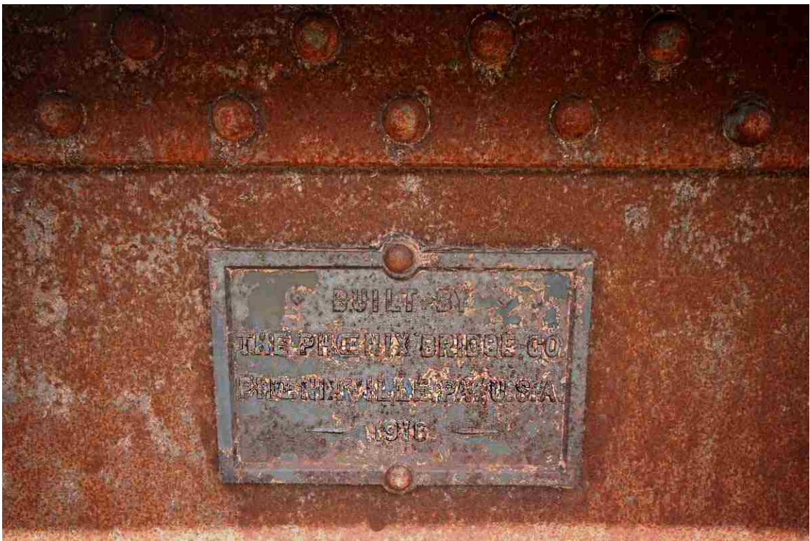
Photo # 88 description: Bridge 145.43, Gorham, "Moose River Bridge No. 1." Builder's plate: "Built by Phoenix Bridge Co., Phoenixville, P.A., U.S.A. 1916." (3 of 3). (fabrication date).
