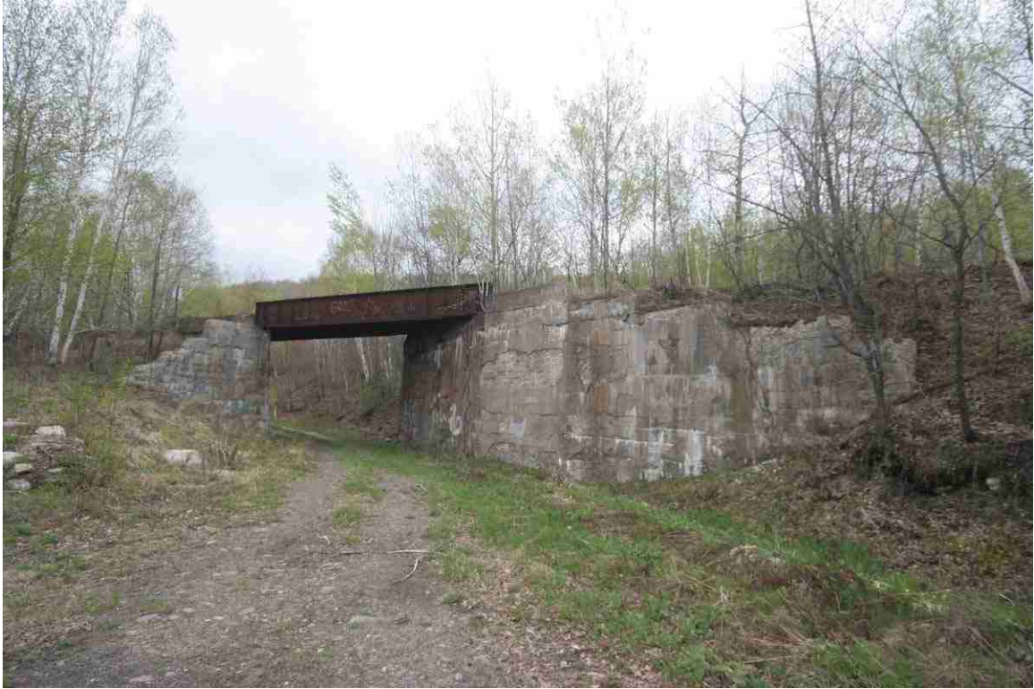
Photo # 131 description: Bridge 153.14 over A&SLRR at Berlin Mills Station, Berlin. West side from former A&SLRR ROW.
