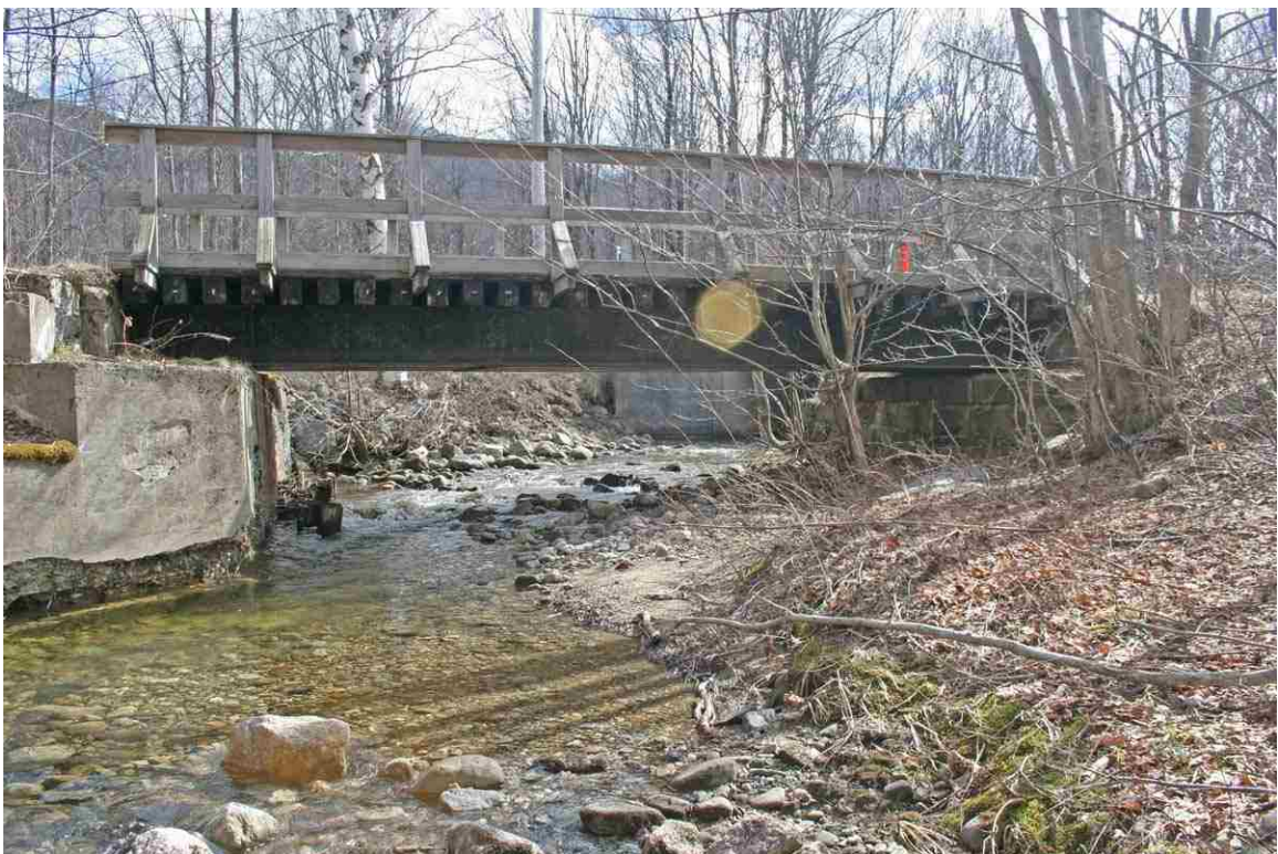
Photo # 76 description: Bridge 144.13 over Bumpus Brook, Randolph. Downstream side showing concrete east abutment. (2 of 2).
