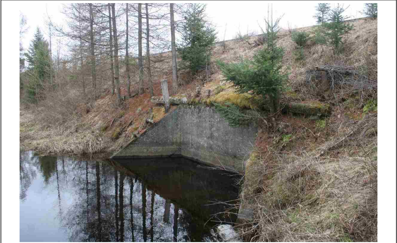
Photo # 5 description: Culvert 129.04, Leonard Brook, Whitefield. Cast iron pipe, 48"; concrete bevel-wing headwalls support high railbed through marsh area along Johns River. Pipe is submerged. 1918.
