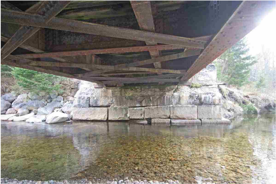
Photo # 45 description: Bridge 138.75 over Israel's R., Randolph. Underside and west abutment showing undermining at south end (left). (3 of 4).
