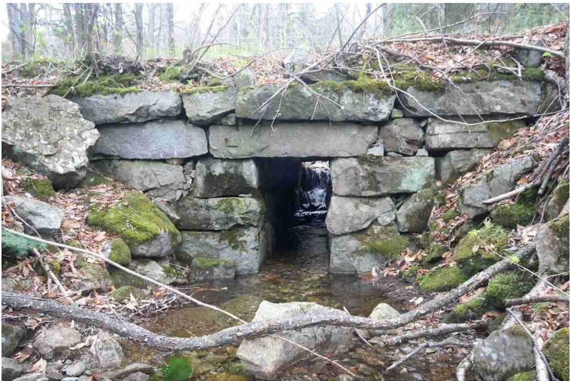
Photo # 54 description: Culvert 141.92, Randolph. Stone box, 36" x 48" tall. Mixed split quarry & fieldstone. nd.
