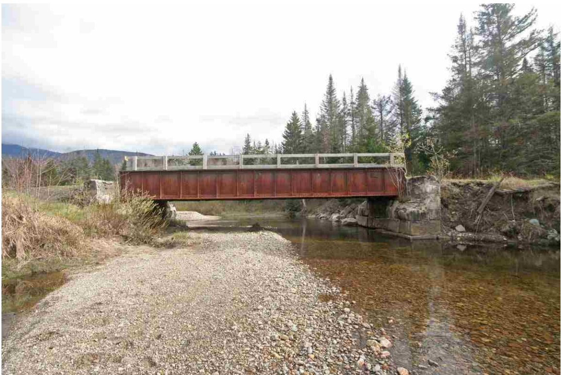
Photo # 44 description: Bridge 138.75 over Israel's R., Randolph. Downstream side. Note washed-out west abutment. (2 of 4).
