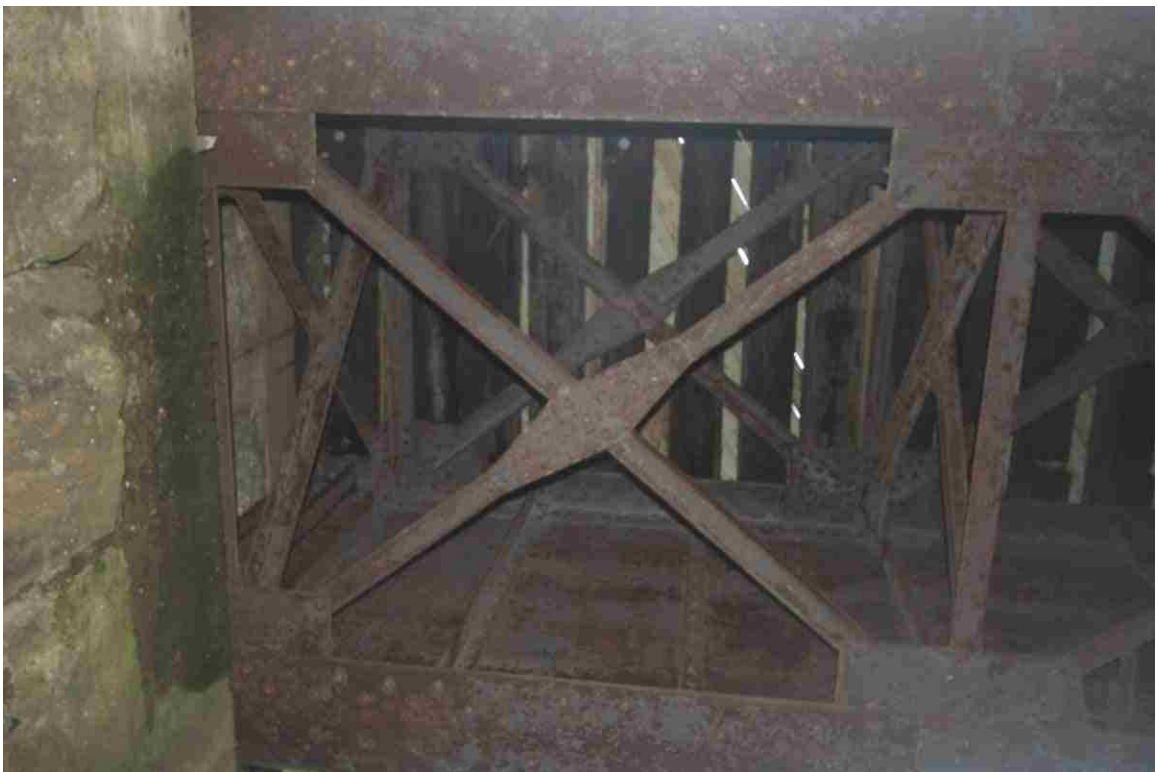
Photo # 106 description: Bridge 146.80, Gorham, "Moose River Bridge No. 3." Underside, view up at west abutment showing deep plate girder and bracing. Note ties in place above under new planking.
