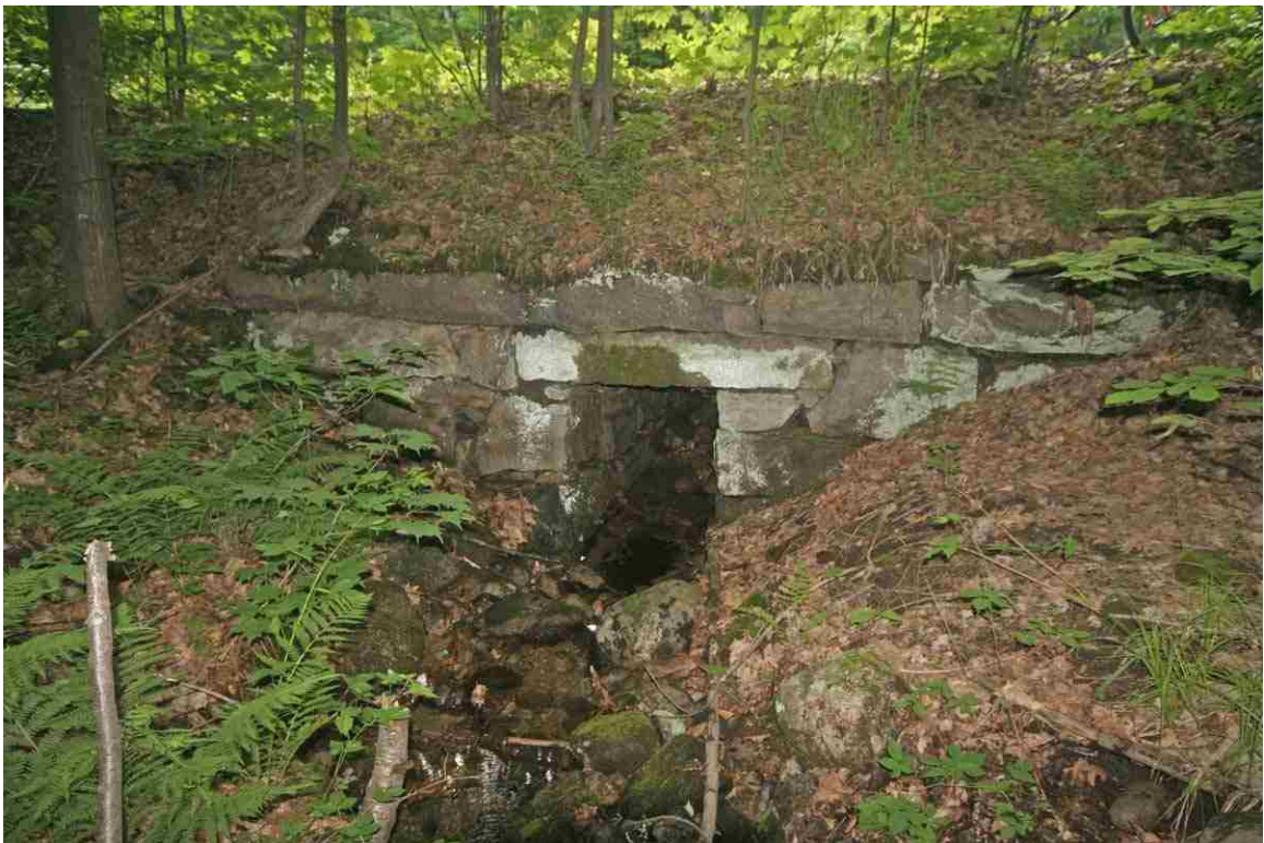
Photo # 126 description: Culvert 151.21, Gorham. Stone box, 4' x 6', mixed split quarry & fieldstone. nd.
