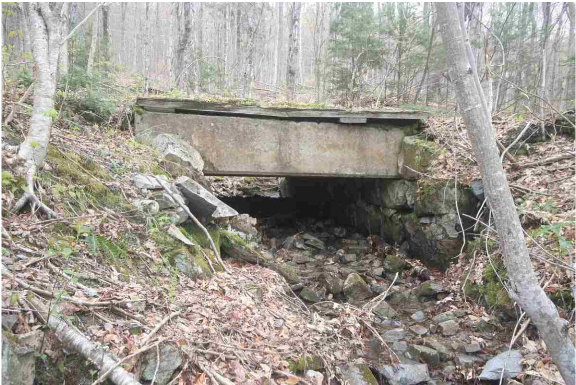
Photo # 52 description: Bridge No. 141.32, over unnamed stream, Randolph. Precast concrete slab, 8' span, on fieldstone walls. Outlet. 1929.
