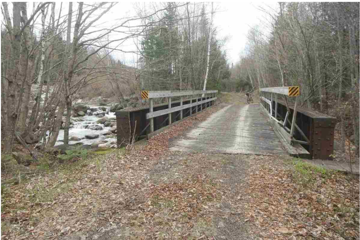
Photo # 60 description: Bridge 142.39 over Cold Brook, Randolph. Thru plate girder, 44' span, on concrete abutments. 1917. (1 of 4).
