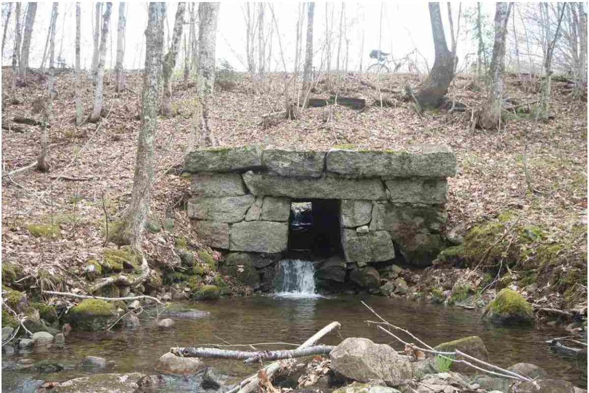
Photo # 56 description: Culvert 142.19, Randolph. Stone box, 36", mixed split quarry & fieldstone. nd. 14' cover. (1 of 2).
