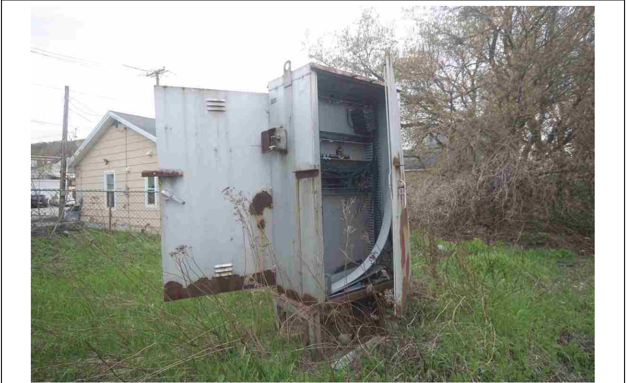
Photo # 137 description: Unity Street crossing, Berlin. Abandoned gate and signal electrical control box. (3 of 3).
