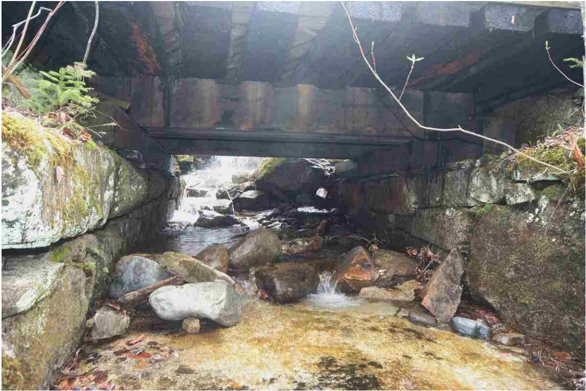
Photo # 99 description: Bridge 146.05, Gorham. Underside and interior from outlet. (3 of 3). Note four massive wood stringers each ~ 8" x 18".
