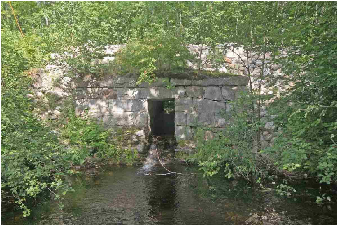
Photo # 124 description: Culvert 150.95, Gorham. Stone box, 4' x 6, split quarry stone. nd. 16' of cover, 40'+ length. (1 of 2).
