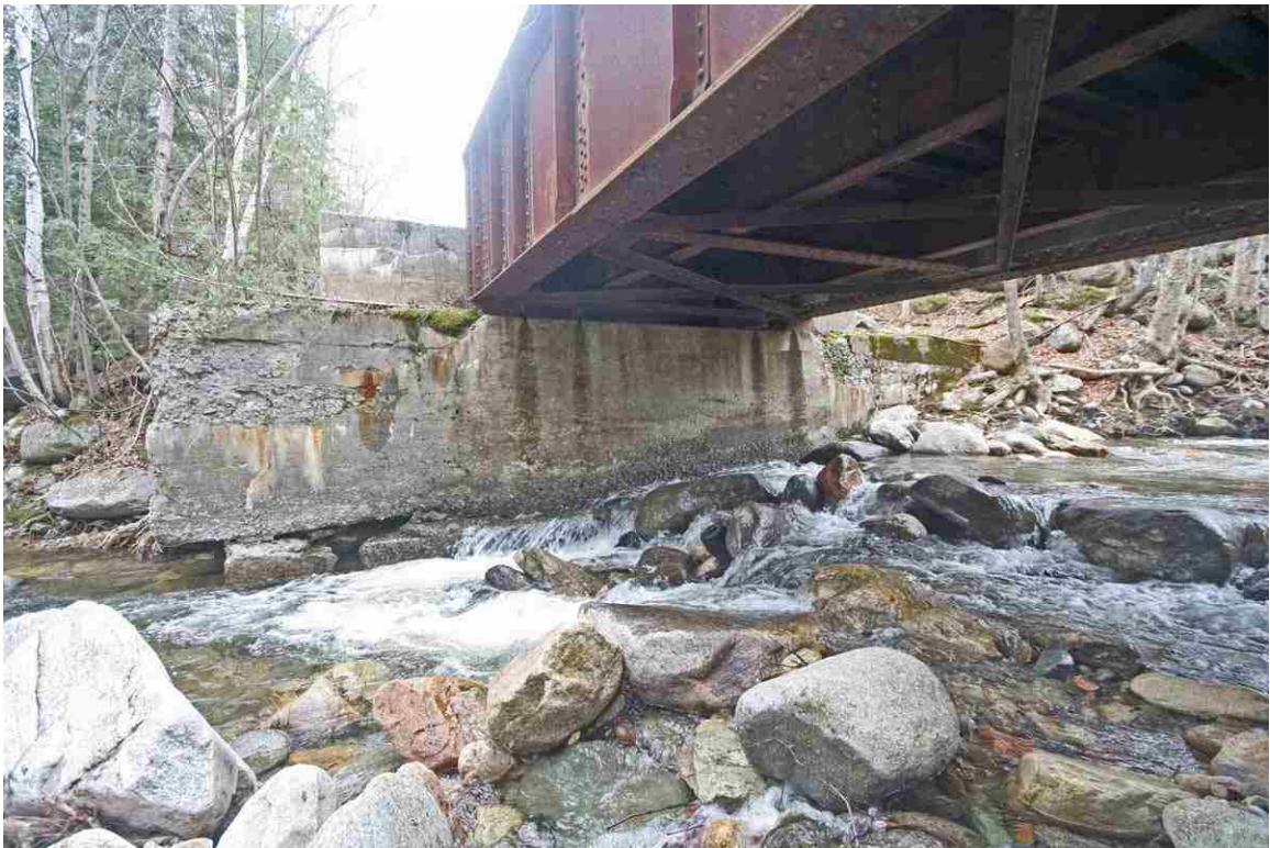
Photo # 62 description: Bridge 142.39 over Cold Brook, Randolph. Underside and east abutment. Note concrete cast on granite footings at left, undermined. (3 of 4).
