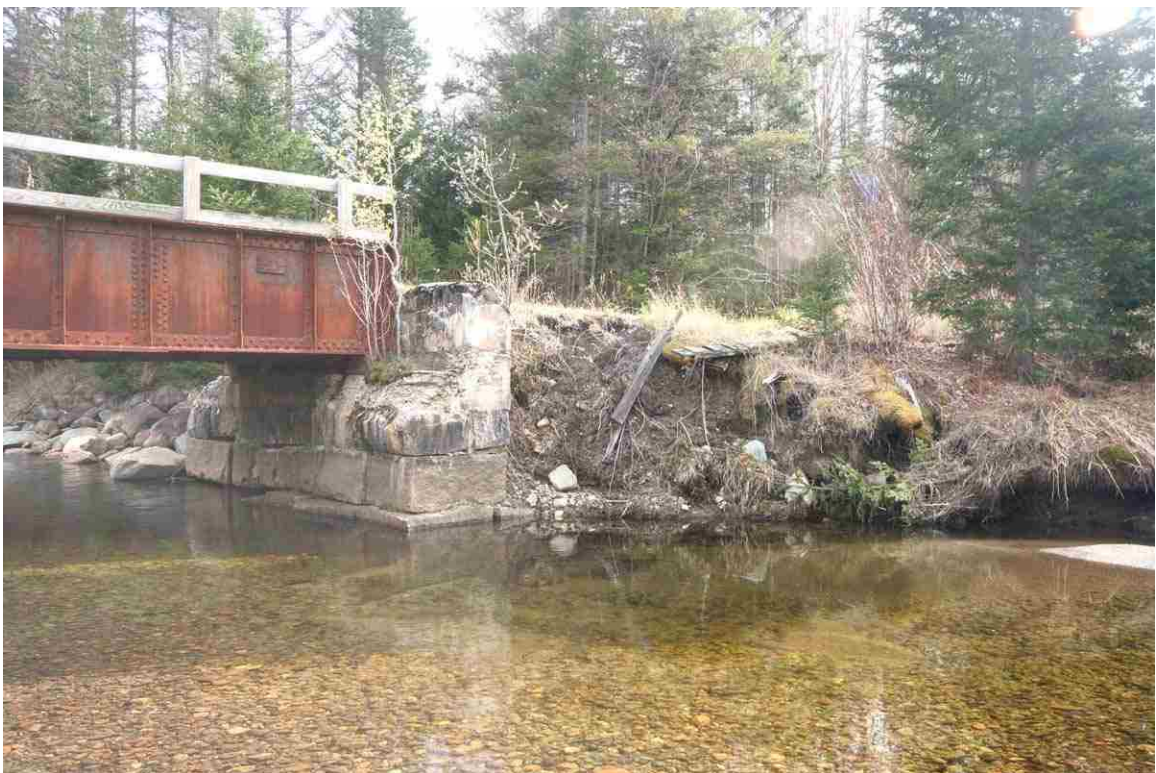
Photo # 46 description: Bridge 138.75 over Israel's R., Randolph. Washout of west abutment, north end. Condition critical. (4 of 4).
