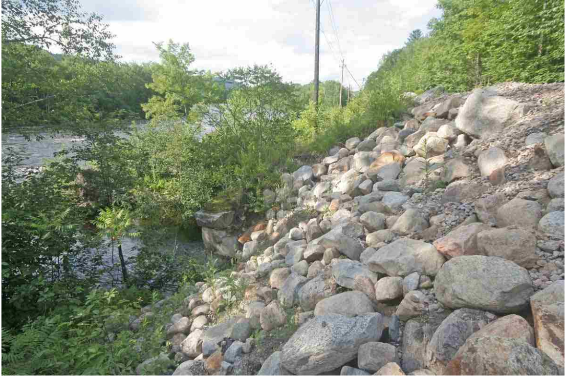
Photo # 125 description: Culvert 150.95, Gorham. Showing extensive fill and rip rap repair to wash out on south side of culvert, visible at center. (2 of 2).
