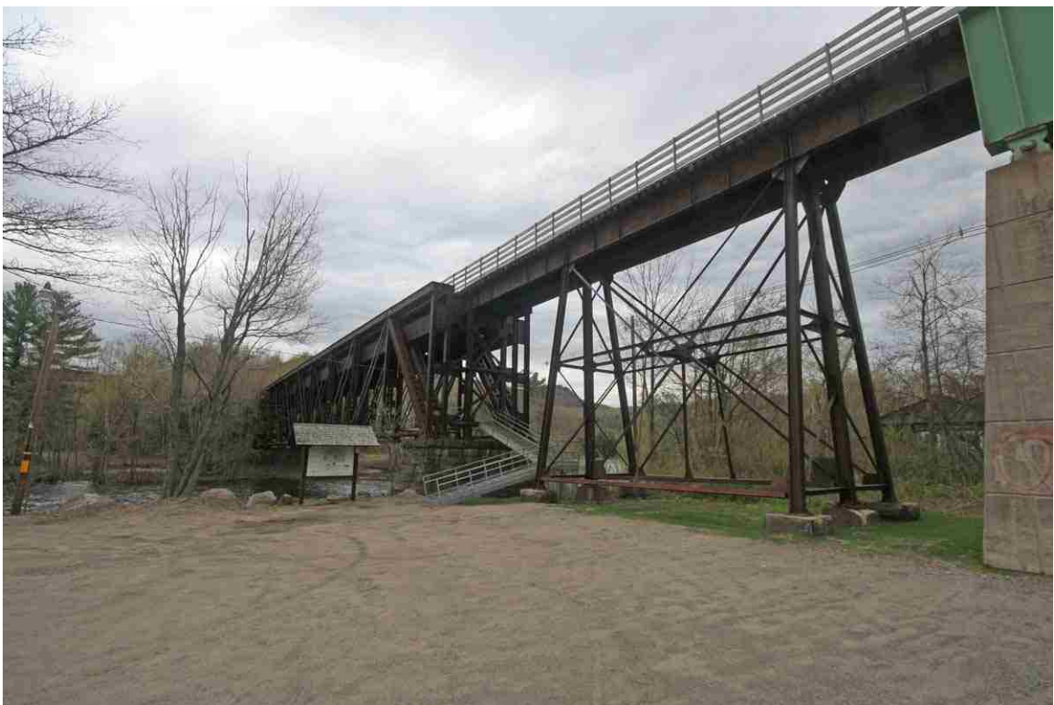
Photo # 118 description: Bridge 149.21, over A&SLRR, NH16, Androscoggin R., Gorham. Deck plate girder spans on steel frame trestle.
