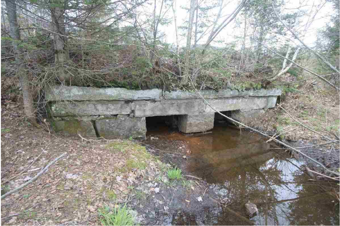
Photo # 47 description: Culvert 140.21, Randolph. Double stone box, 48", quarry-split stone. nd. Rare and outstanding example of double box. Outlet. (1 of 2).
