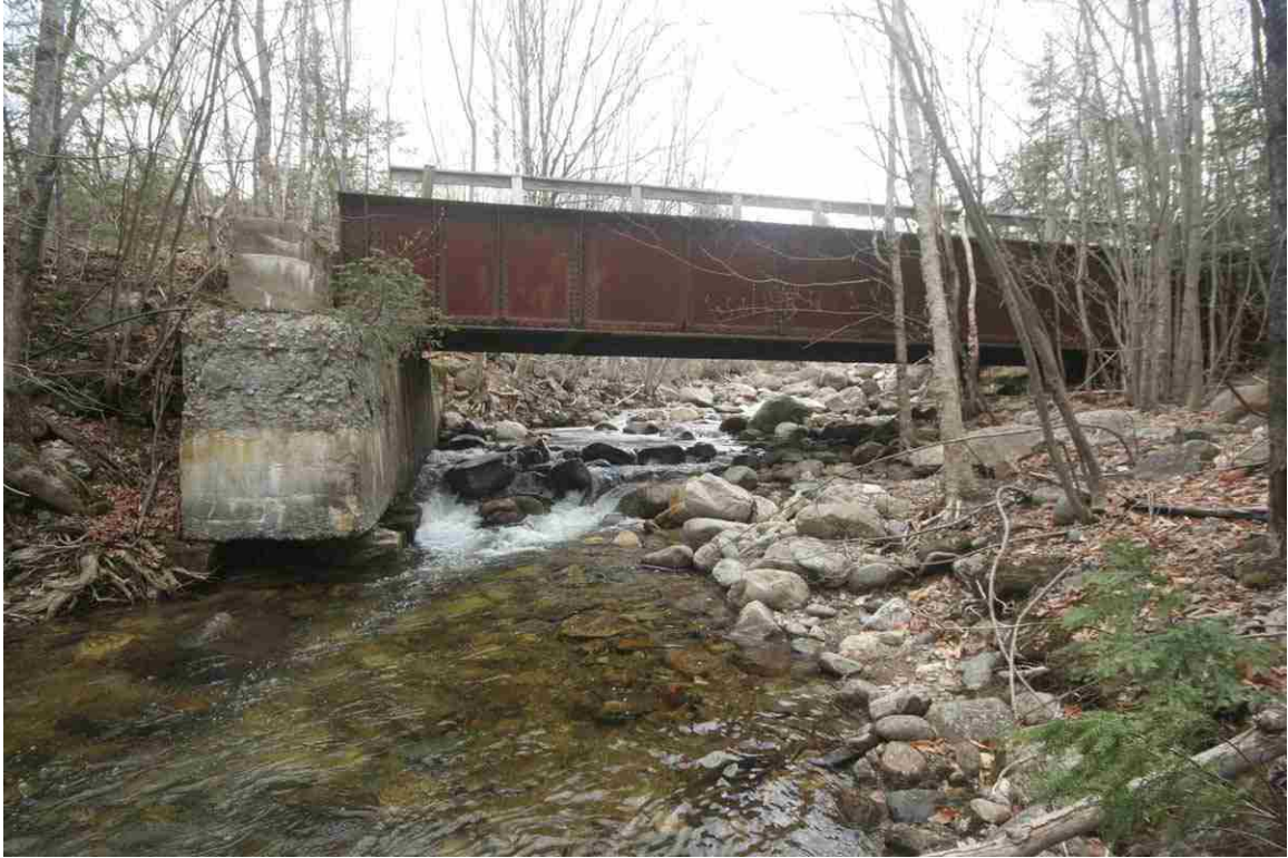
Photo # 63 description: Bridge 142.39 over Cold Brook, Randolph. Downstream side, showing critical undermining of north end of east abutment. (4 of 4).
