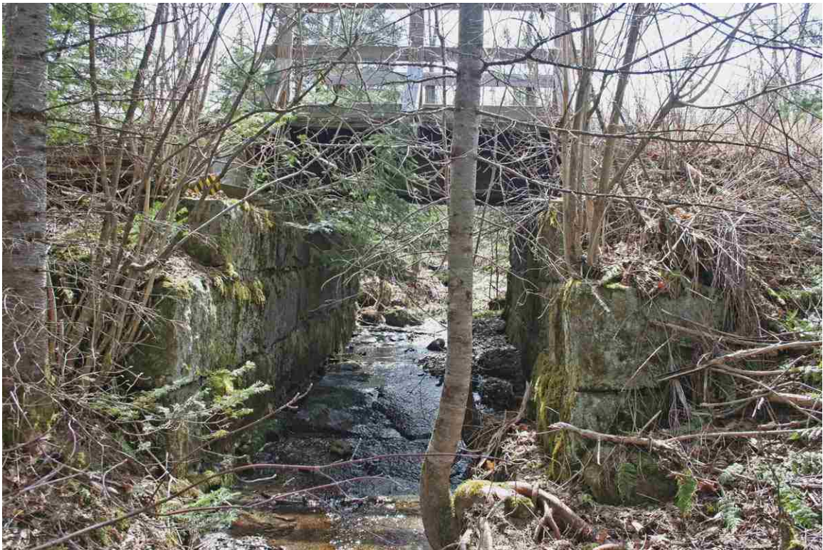
Photo # 30 description: Bridge 136.56 over unnamed stream, Jefferson. Wood stringer, 8' span on split stone abutments. 1928.
