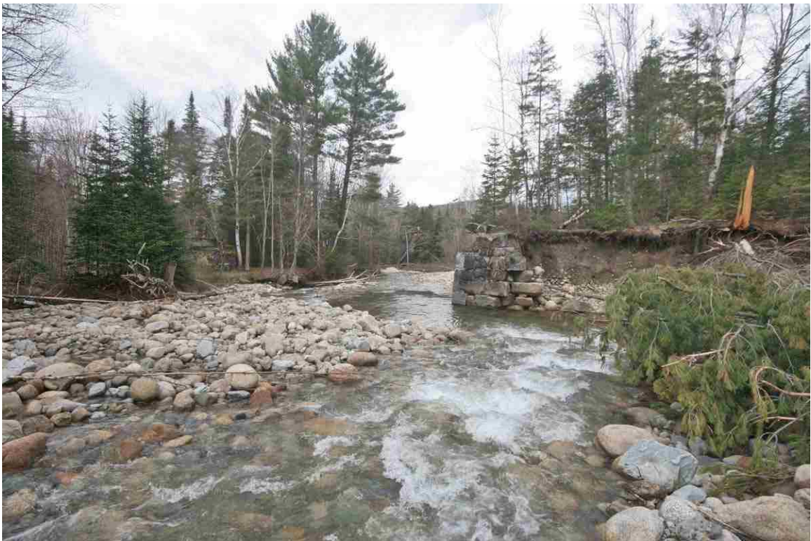
Photo # 36 description: Site of Little River Bridge, Carroll. mp~128.12. Bridge type unknown. Stone abutments left on both banks. East abutment washout and collapsing. (1 of 4).
