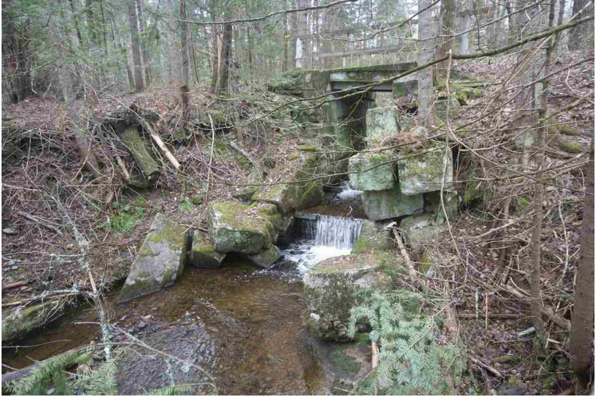
Photo # 45 description: Bridge 128.93 over unnamed stream, Carroll. Downstream side. Collapsing. (2 of 2).
