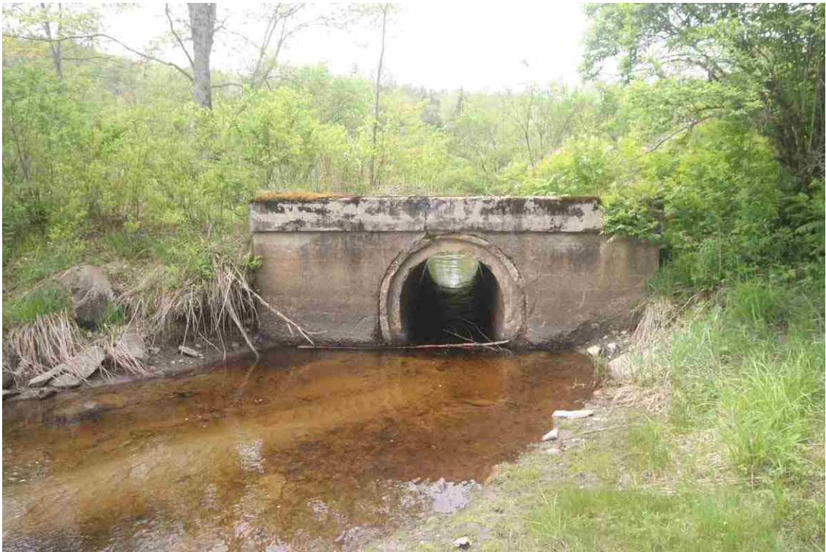
Photo # 11 description: Culvert 128.38, Dalton. Concrete pipe, 36" with concrete headwalls. nd. Present in 1914; replaced a wood stringer span.
