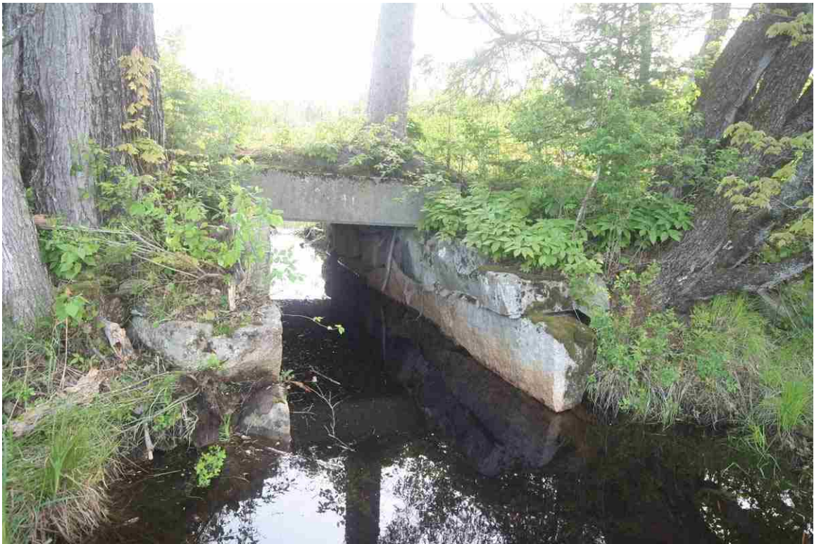
Photo # 23 description: Bridge 129.13 over unnamed stream, Dalton. Concrete slab, ~5' span, on split quarry and fieldstone abutments. nd.
