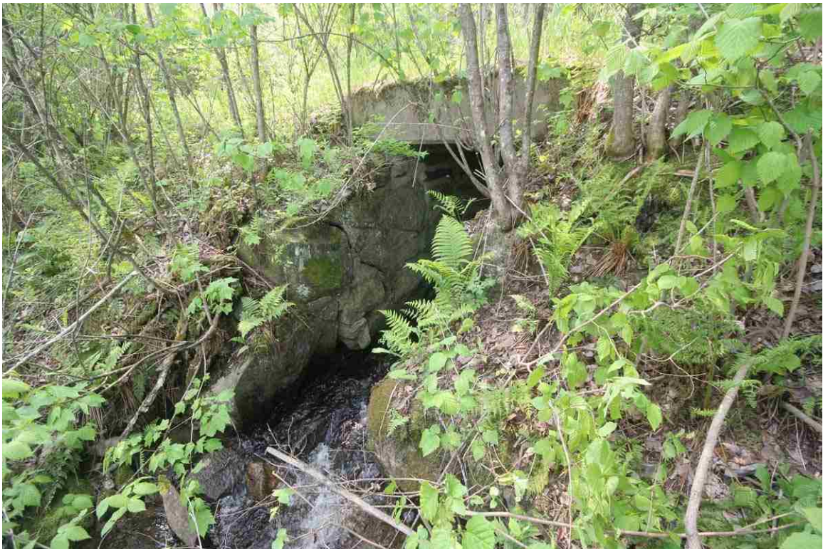
Photo # 2 description: Bridge 126.81, over unnamed stream, Dalton. Concrete slab, 4' span, on split fieldstone abutments. nd. Downstream side. (1 of 2).
