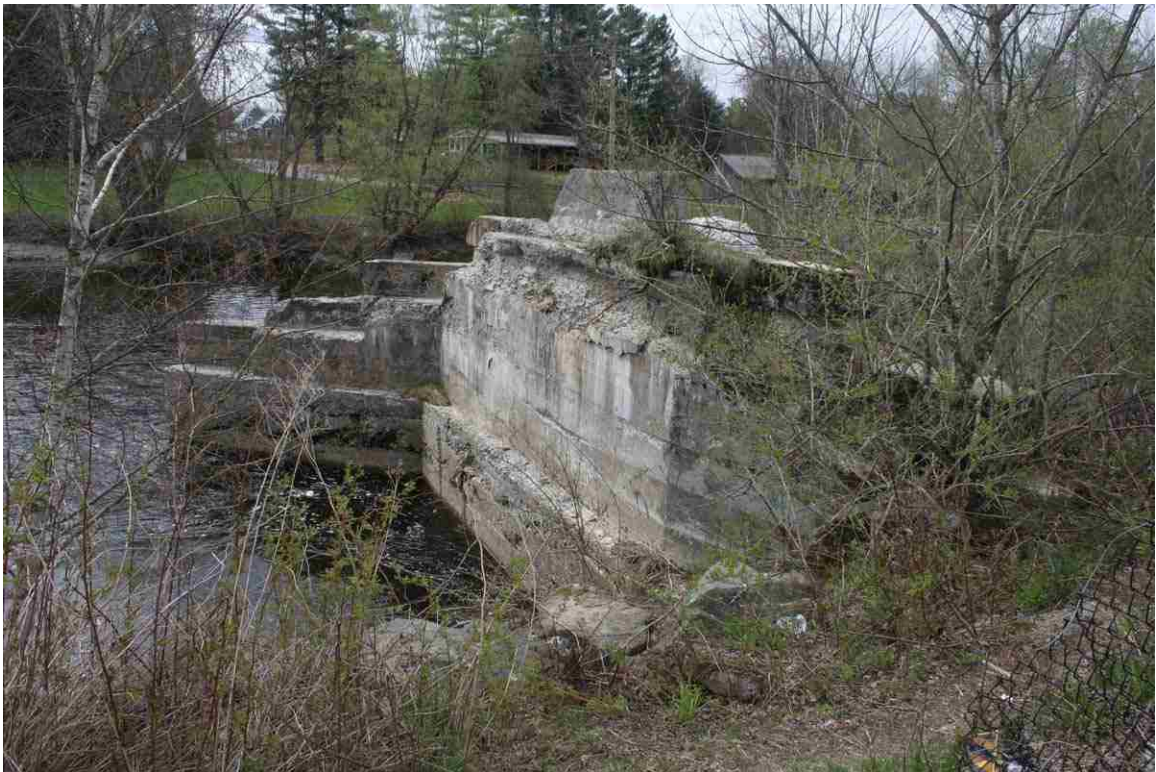
Photo # 40 description: North abutment of B&M Bridge 136.01, showing exposed back side, the railbed fill completely washed out. Provides interesting look at construction methods.
