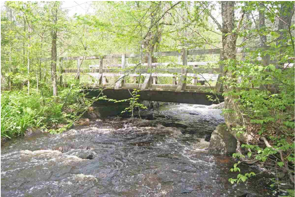
Photo # 19 description: Snowmobile Bridge over unnamed stream, mp~128.75, Dalton. Improvised steel stringer bridge on split fieldstone abutments. nd.
