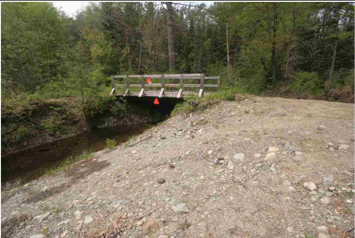
Photo # 8 description: Snowmobile Bridge, over unnamed stream, mp 127.78, Dalton. Modern steel stringer on treated wood bearings. Apparently replaced 12" pipe culvert formerly at this location.
