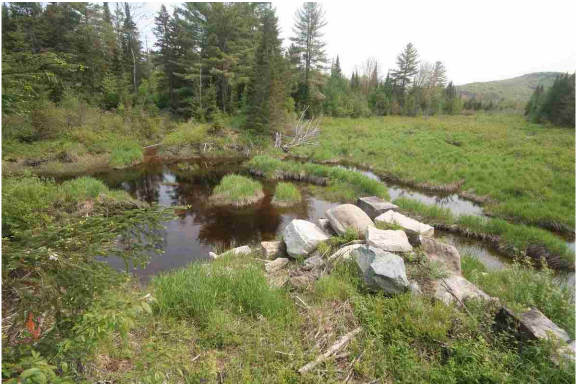
Photo # 30 description: Character of ROW/Trail at mp~131.01, Lancaster. Location of 48" concrete pipe culvert, washed out. Trail detours west over snowmobile bridge and rejoins ROW 500' north.
