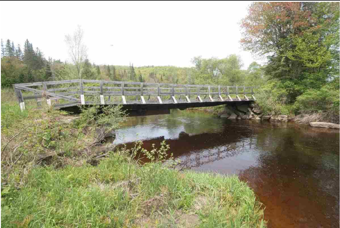
Photo # 6 description: Snowmobile Bridge over Johns R., Dalton. mp 127.45. Modern improvised steel I-beam stringer for trail use replaced covered wood truss. Repaired/reconstructed stone abutments. nd.
