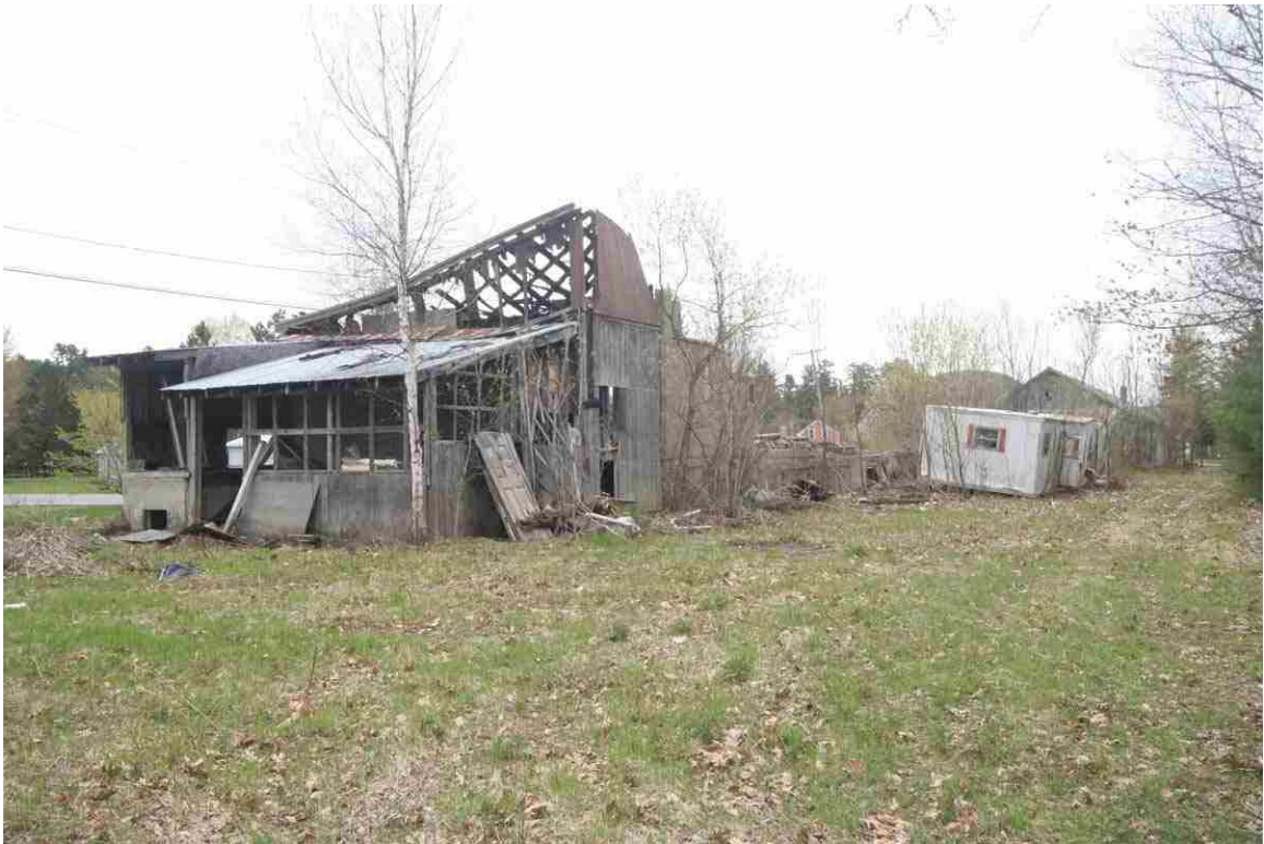
Photo # 52 description: Remains of depot buildings along Depot St., Lancaster. ~mp 136.78. Photo from center of former ROW, looking south.
