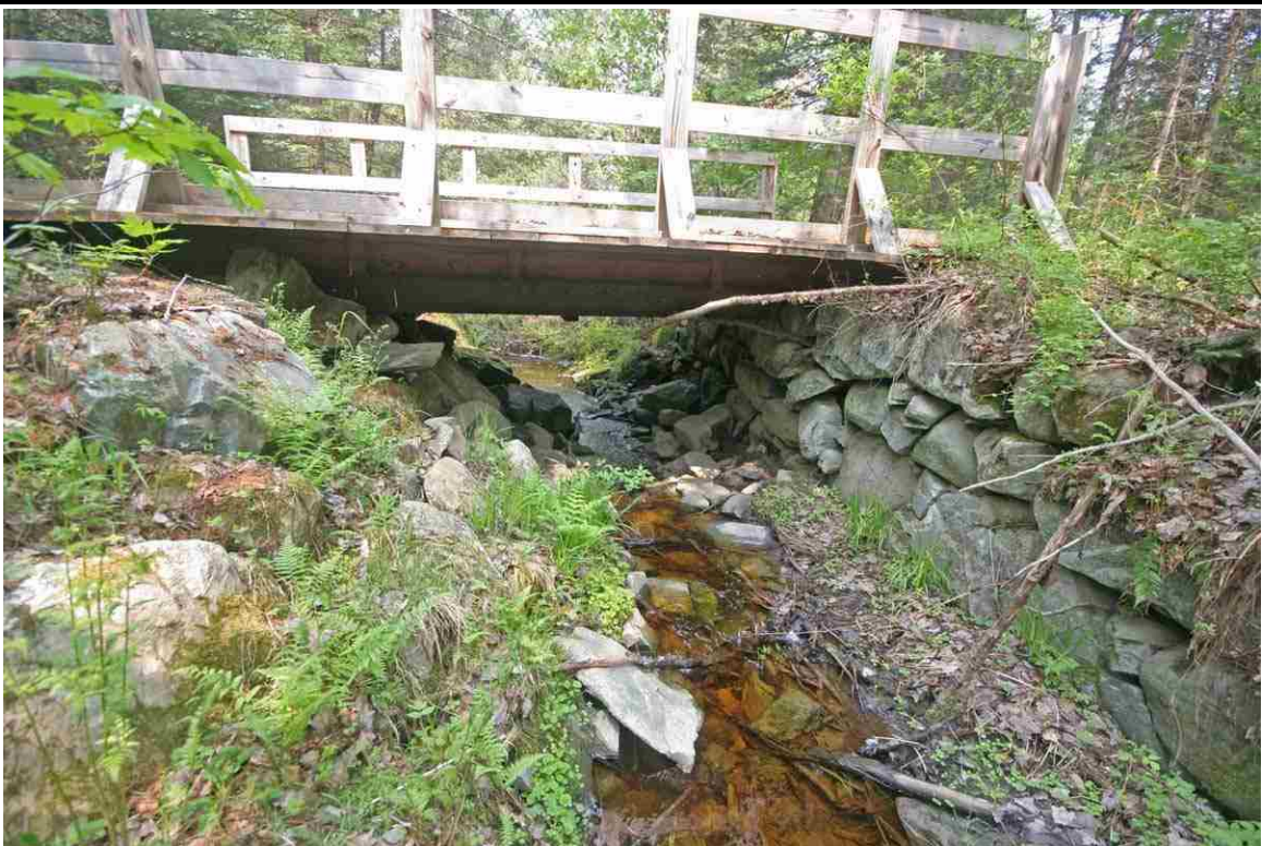
Photo # 28 description: Snowmobile Bridge over unnamed stream, mp~130.45, Dalton. Treated timber stringer on reconstructed fieldstone abutments.
