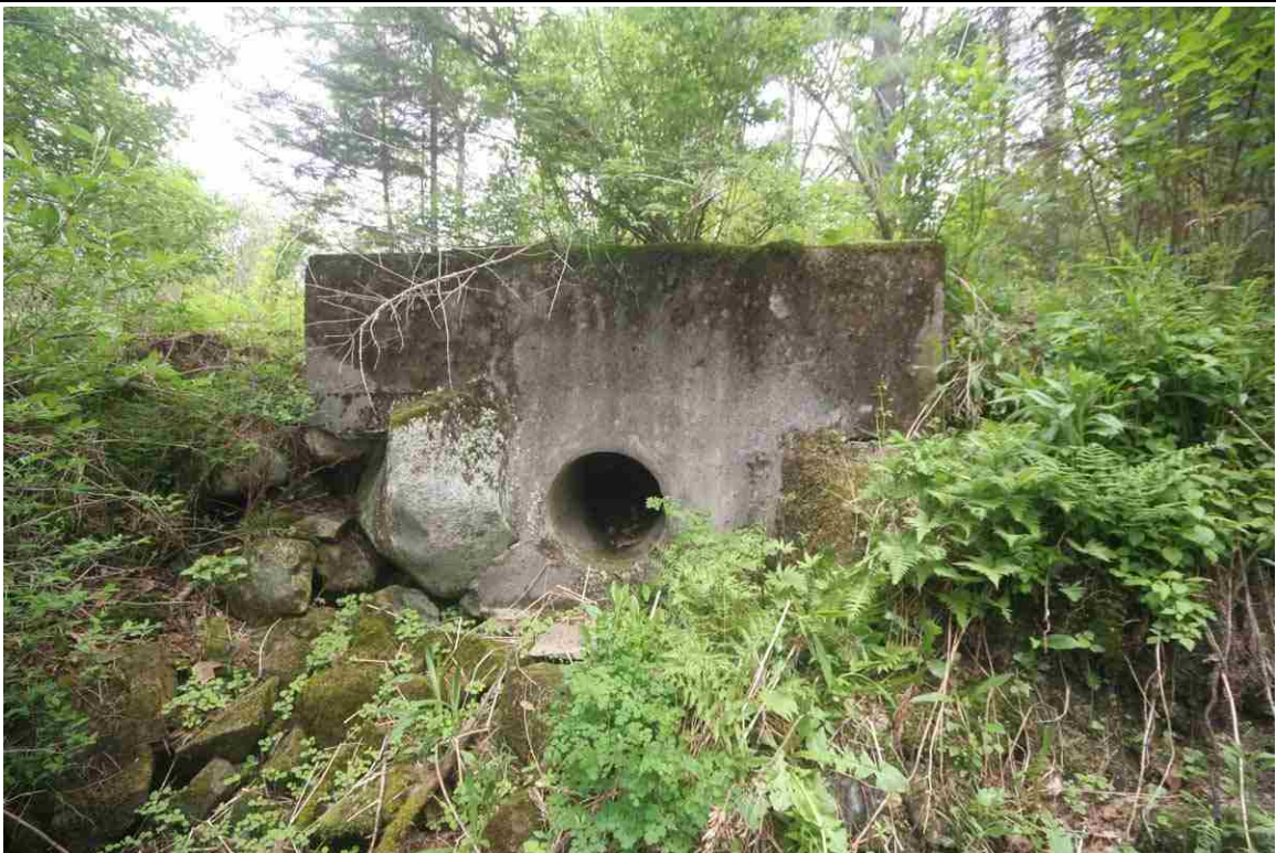
Photo # 14 description: Culvert 128.45, Dalton. Cast iron pipe, 18" with concrete headwalls. nd. Appears to have replaced a stone box culvert previously at this location.
