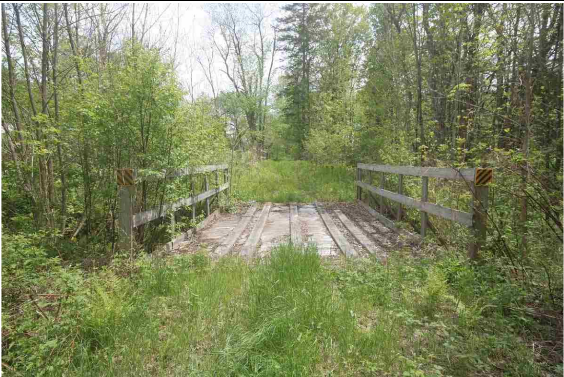
Photo # 20 description: Snowmobile Bridge over unnamed stream, mp~128.76, Dalton. Improvised steel stringer on split fieldstone abutments. nd.
