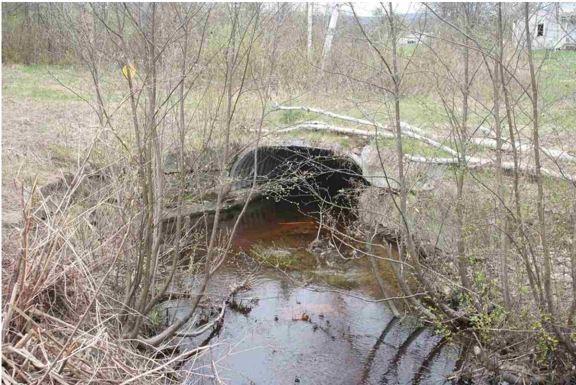
Photo # 56 description: Metal arch culvert carrying ROW over unnamed stream near Kilkenny St., Lancaster. ~mp 136.84. Stone walls possible remains of box culvert.
