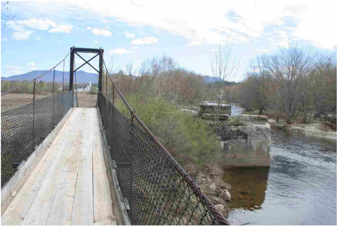
Photo # 39 description: Israel R. snowmobile suspension bridge at foot of of Heath St. Lancaster. North abutment of B&M Bridge 136.01, concrete, at right.
