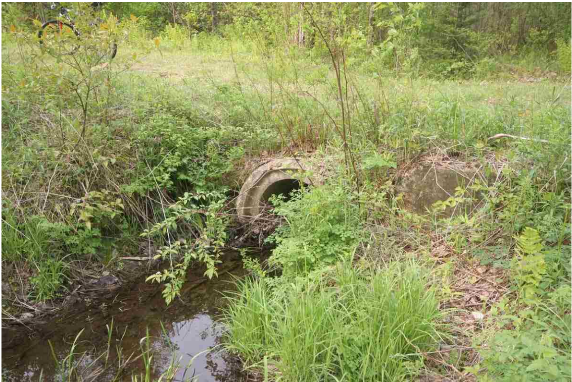
Photo # 24 description: Culvert, mp~129.50, Dalton. Akron pipe, 38". Small section of presumed concrete headwall is visible; remaining wall missing or buried. nd.
